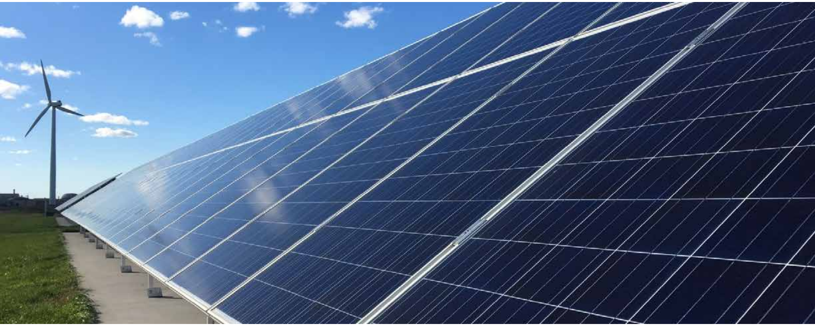
All images: Moorhead Public Service solar and wind generation site
